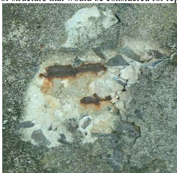
Figure 8: Spalling and cracking of concrete due to carbonation-induced corrosion on parapet walls at the Menzies site.
