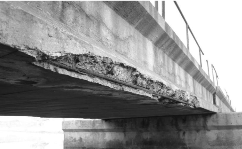
Figure 1: Corrosion-induced damage on a concrete bridge exposed to air-borne chlorides close to the shore in Cape Town
