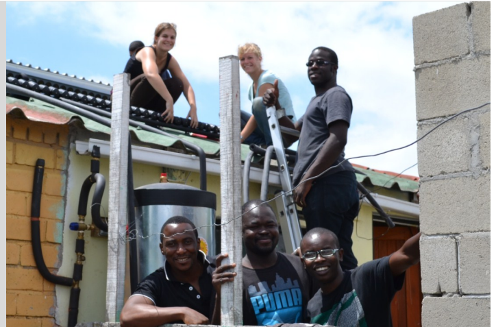
Verena Steub, Helena Hingerl (from Crossing Borders in Germany); David Oyedokun, Tshina Mulumba, Roaldje Nadjiasngar and Blessing Katsande (IEEE student members) busy installing the 300 litre solar geyser
